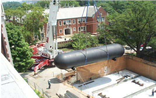
NEW 30 000-GALLON PROPANE TANK
