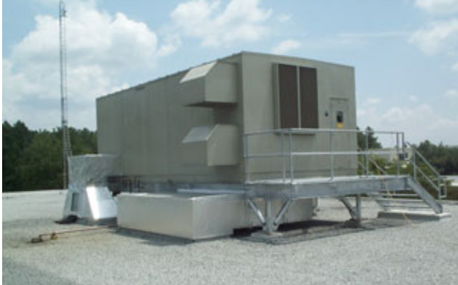
AIR HANDLING UNIT
