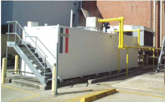
10,000-GALLON FUEL STORAGE TANK
